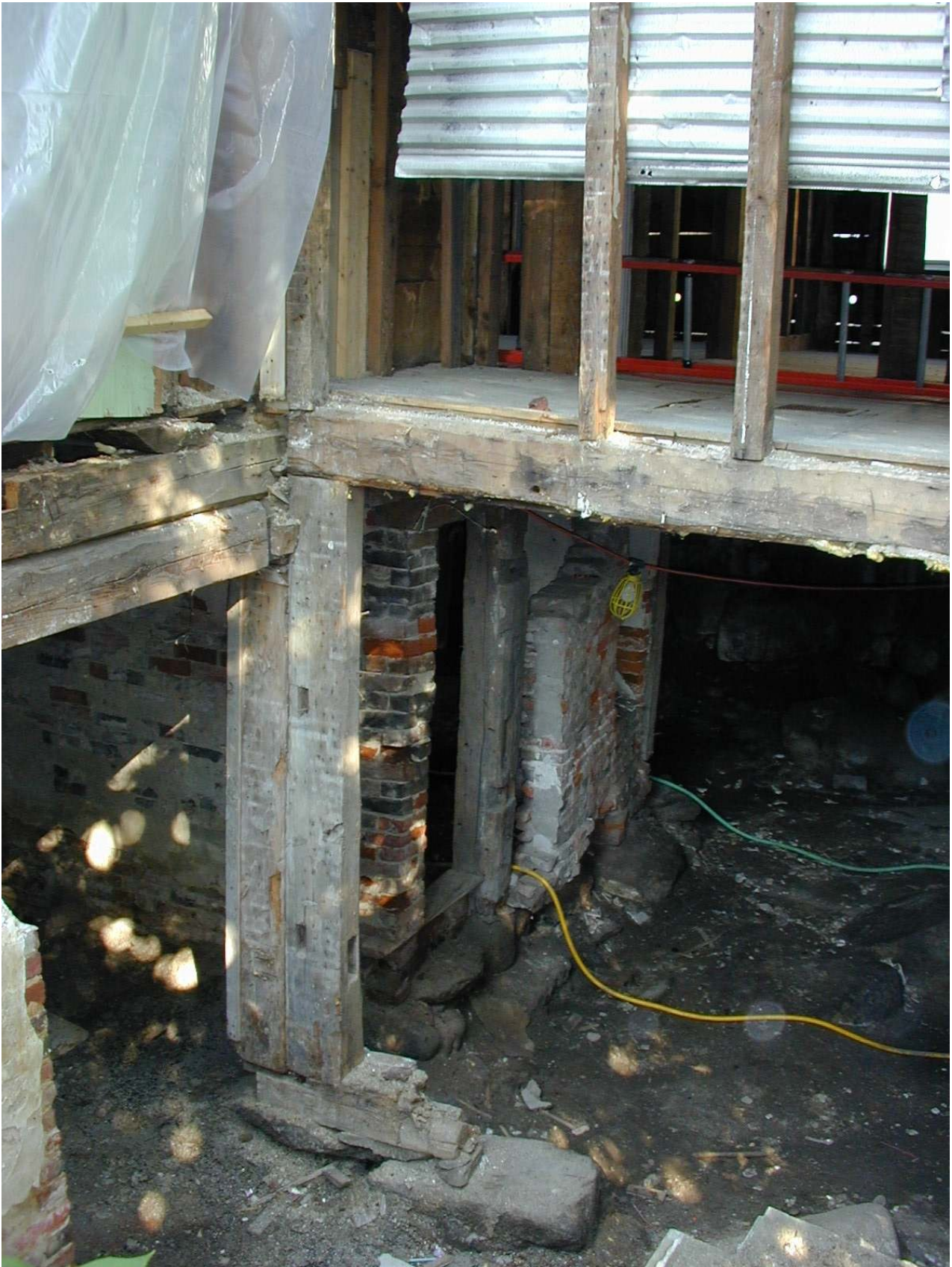
(A.) View of rear of #925 showing re-used timbers shoring up floor.
