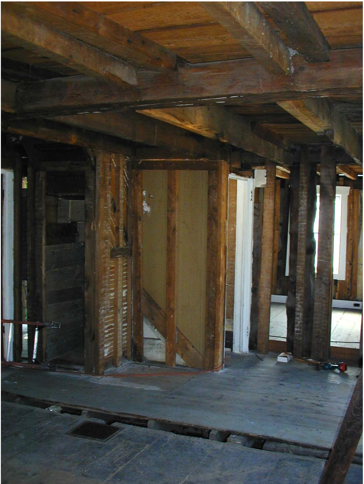
(C.) View through the front portion of #925 showing timber frame ceiling and joins in floor.
